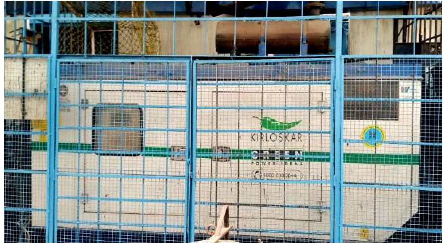
24x7 Generator facility
