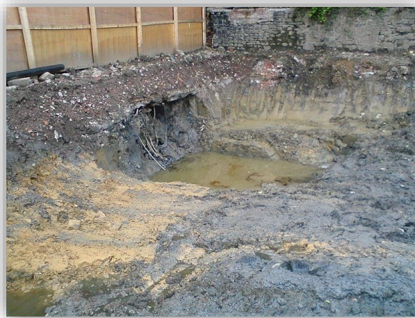
Excavation showing soil contamination at a disused gasworks in England
